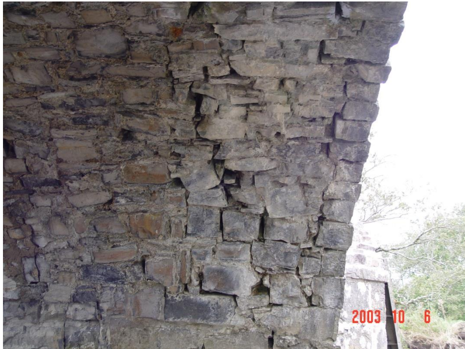
Diagonal and vertical cracks and external ring separation
